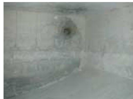
Typical appearance after three years arduous use – almost unchanged since installation
